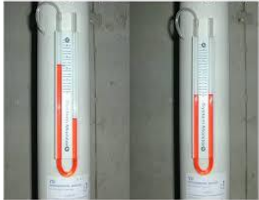
Photos courtesy of VSI Radon Reduction Corp
